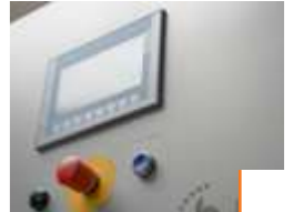
Digital control panel
